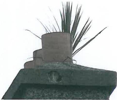
Cracked chimney pots and vegetation to top of stack. Cracked/damaged render to top section.
