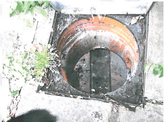
Obstructions to below ground drainage system.
