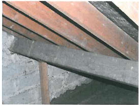
Woodworm evident to roof purlin.
