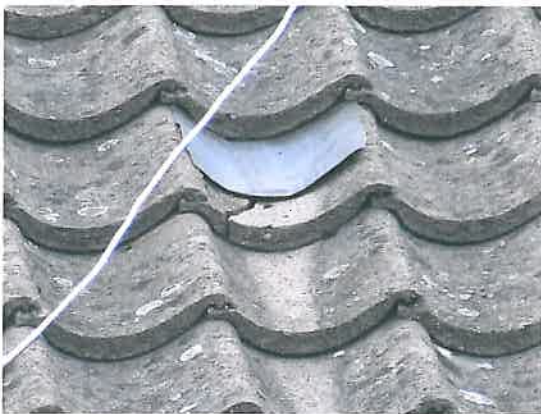
Cracked roof tile to rear roof slope.
